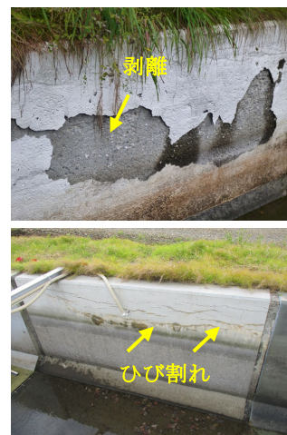
Fig.1 補修材の早期劣化の事例 Typical early deterioration of repair mortar
